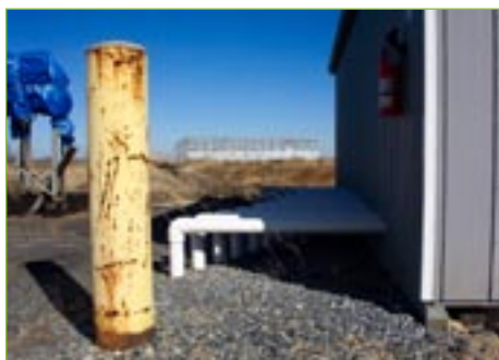
The air sparging system, which works in conjunction with soil vapor extraction, was activated in October 2004.
